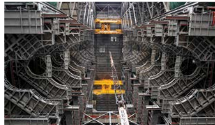
Final work platform installed in Vehicle Assembly Building for Space Launch System. (NASA/Frank Michaux)
